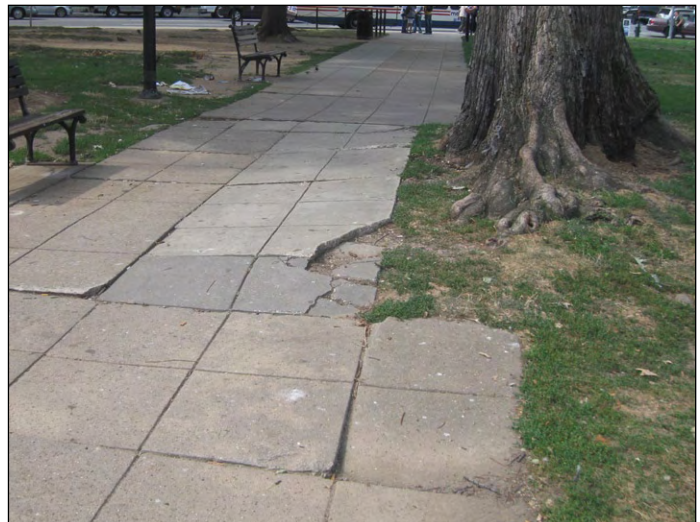
In compacted soil, tree roots often grow in the small void space just beneath the pavement, causing sidewalk heaving.
